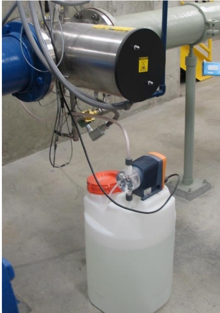
Example of the Pressurized Ultra Wipe® chemical storage and distribution pump as a new system is being installed.
